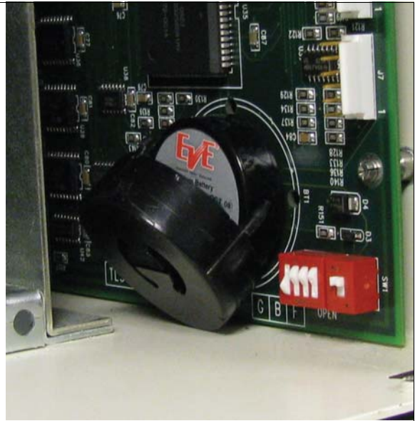
B. Battery Cover Dislodged
